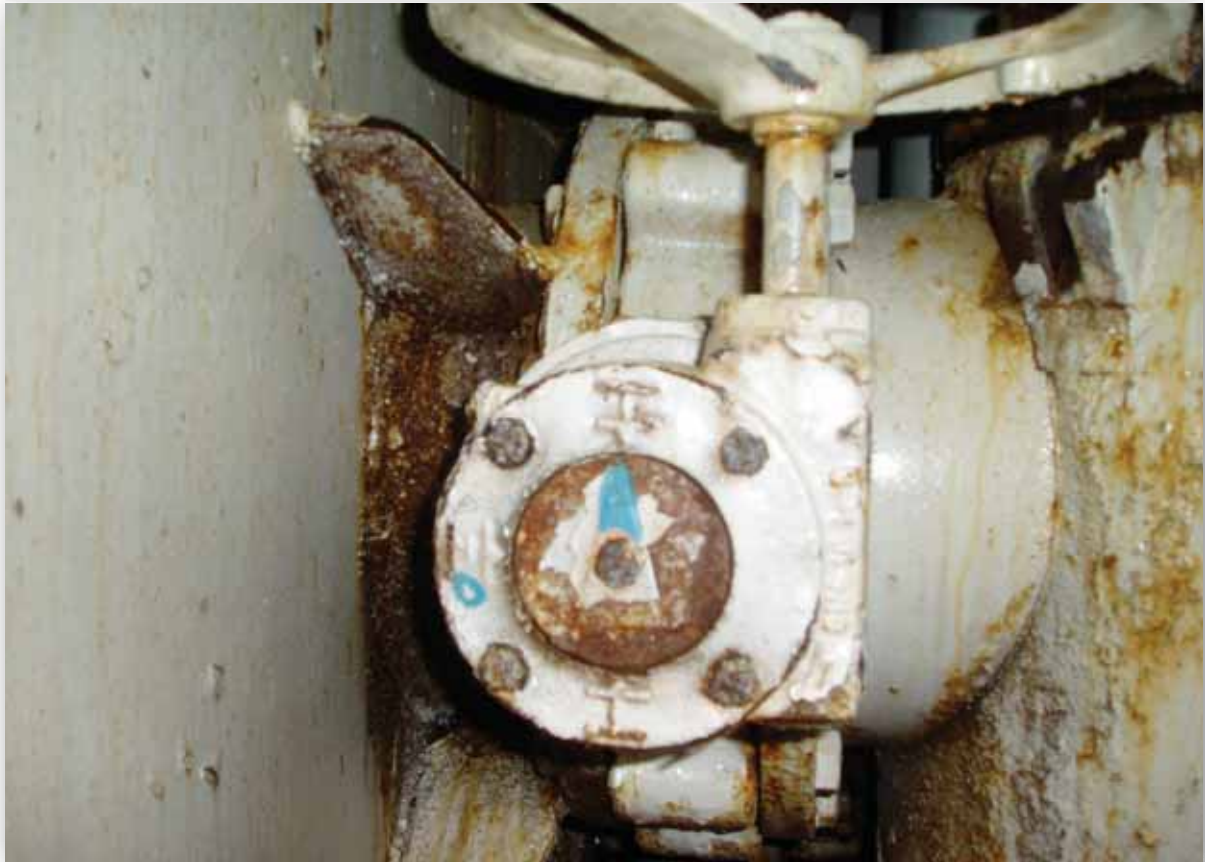
Appendix 8.4.2 Photograph of valve position indicator
