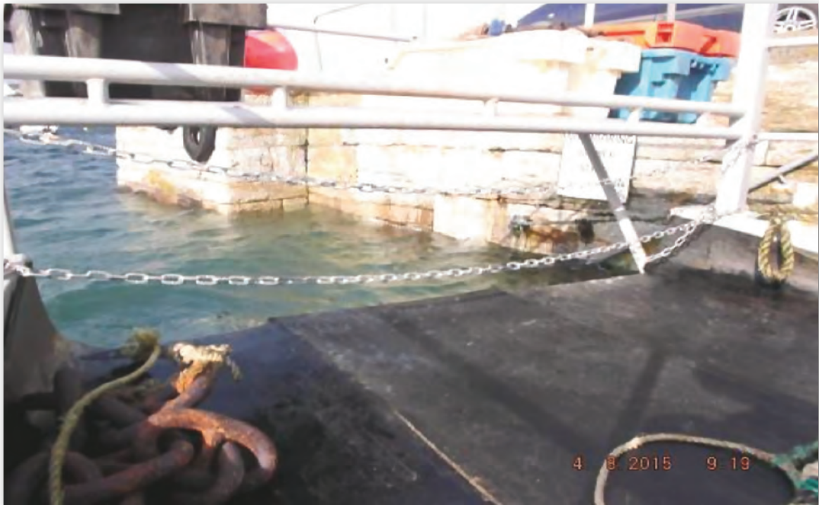
Photograph No. 3 - Stern area from deck level showing removed bulwark
